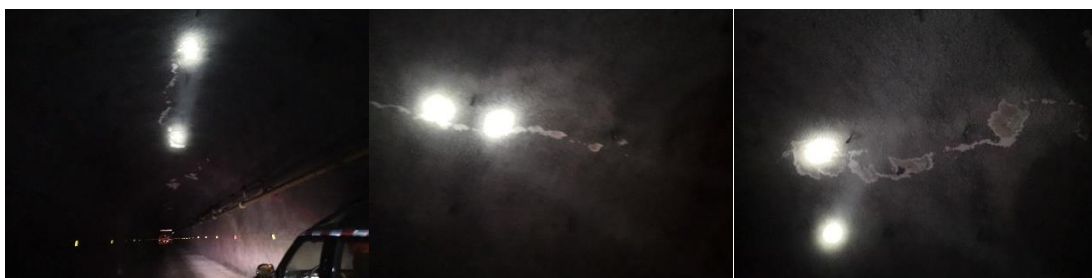
Fig. 4.1 Picture of concrete slagging in the roof of the roadway
