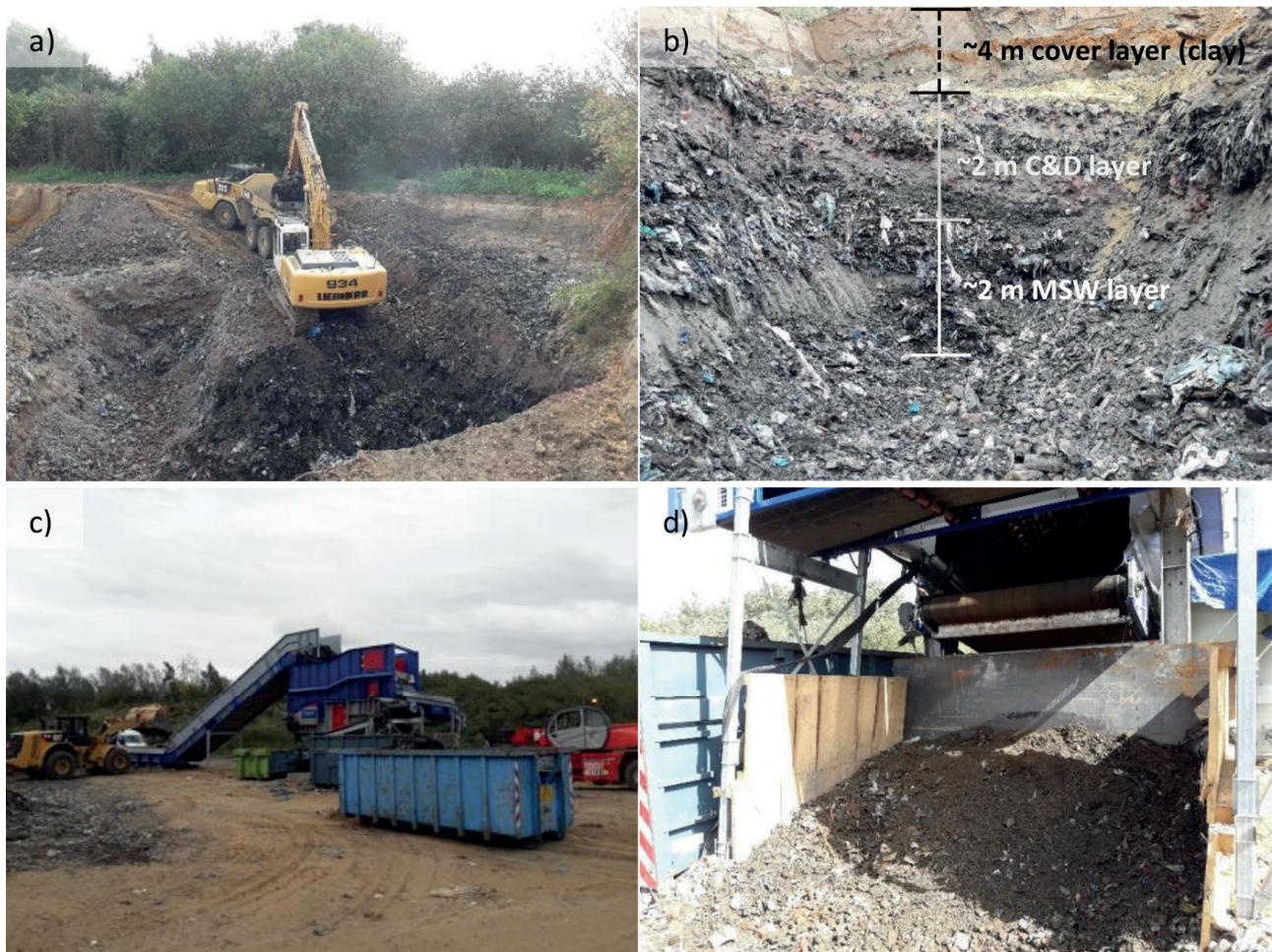
FIGURE 2: a) Material excavation, b) excavation volume, c) ballistic separator and d) fine fractions.
