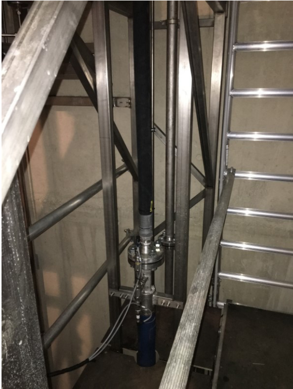
Figure 63: Pump discharge (REDA D2100EZ)
