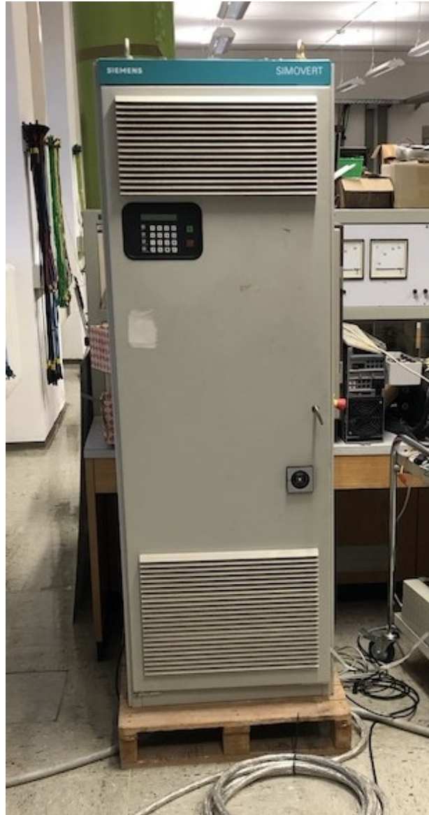
Figure 15 VSD Drive SIMOVERT P
