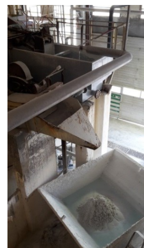
Figure 6: Sand separator II
