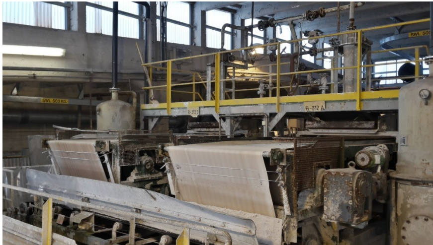
Figure 9: Band filter and dewatering cyclones
