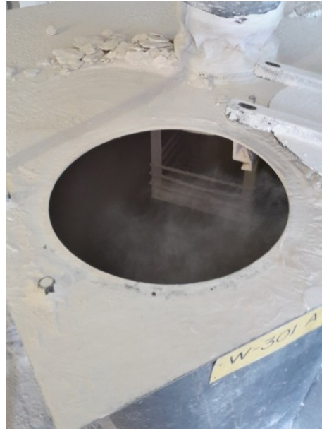
Figure 21: Sampling point 4 DOLIME silo II
