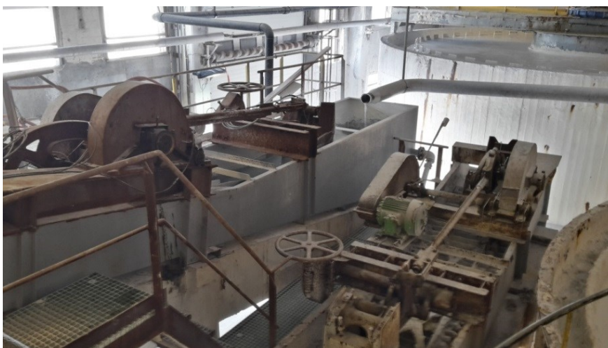
Figure 5: Sand separator I/ rake classifier
