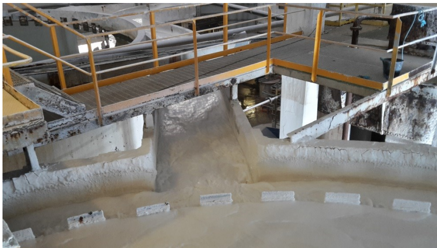
Figure 4: Overflow hydro separator
