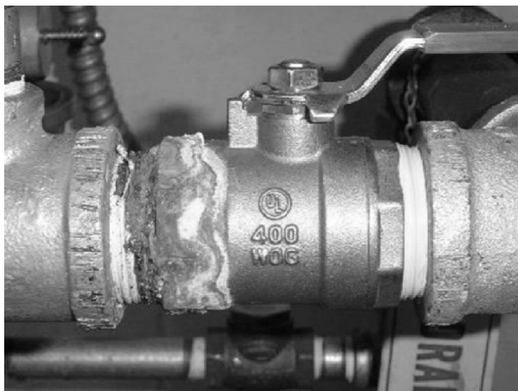
Figure 5-2 Galvanic corrosion of galvanized piping in connection with bronze valve[31]
