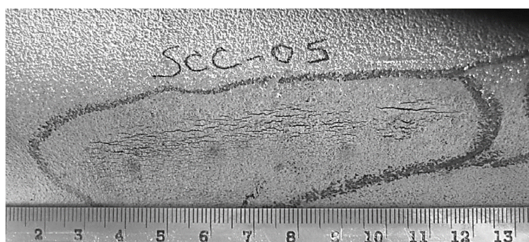
Figure 5-8 Clustered "colonies" of SCC on the outside of a carbon steel Pipeline[31]
