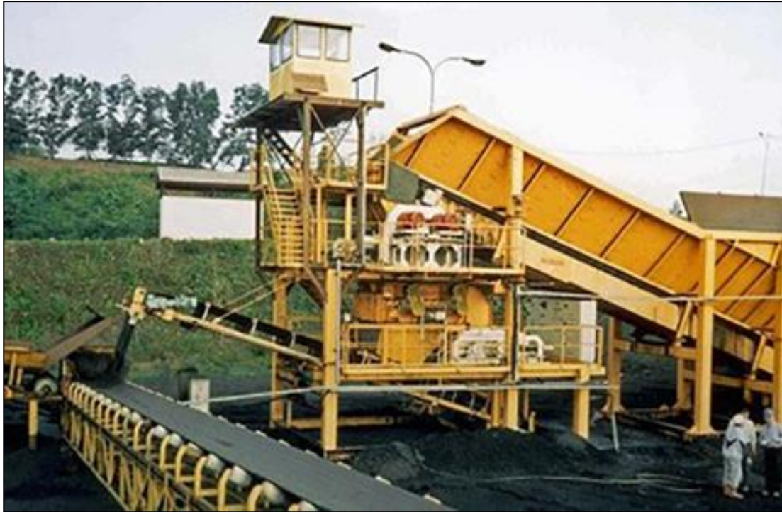
Figure 9: Fixed In-Pit Crusher Station of FLSmidth [5]
