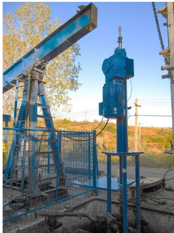
Figure 10: Installed LRP from Asset 9 Moldava Sud
