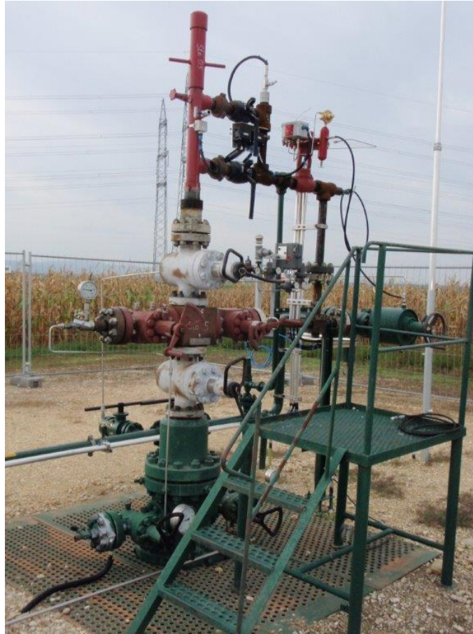
Figure 62: Plunger lift surface equipment - Well 2
