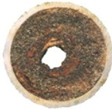
Figure 4: Wax deposit in a pipe
