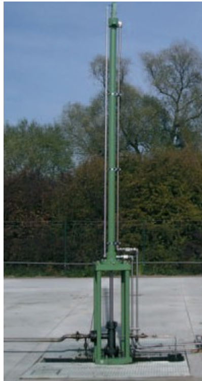
Figure 13: Hydraulic Cylinder on Wellhead, Landau [17]
