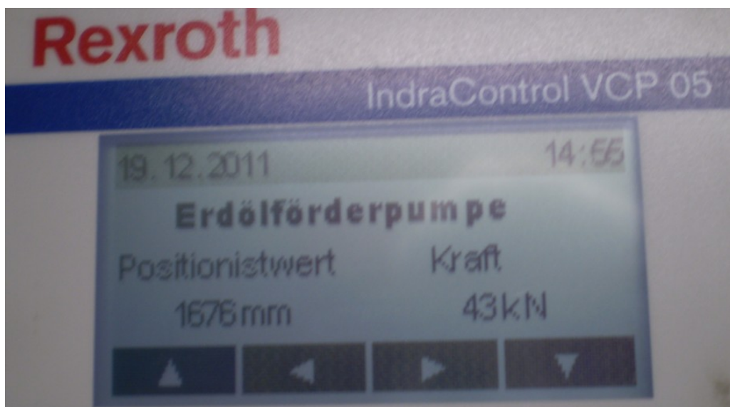
Figure 18: Display of the control station[1]
