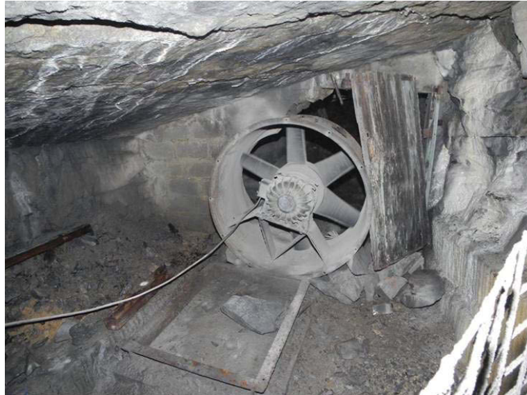
Figure 170: Fan at the weather shaft
