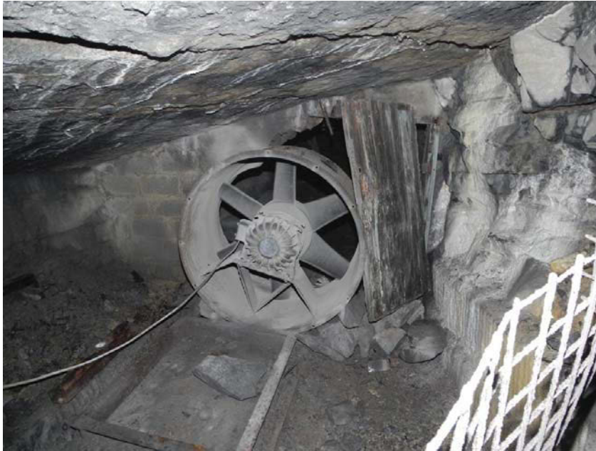
Figure 36: Ventilator, at weather shaft
