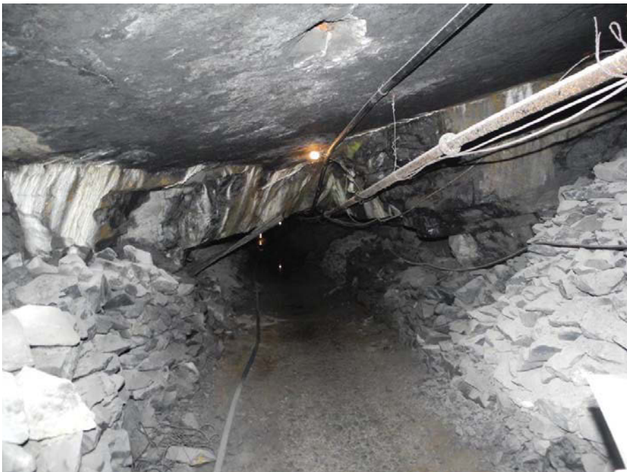
Figure 24: Major fault „inside“; photo number: 1427
