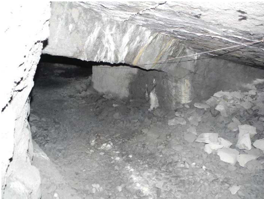
Figure 22: Major fault „inside“; photo number: 1738
