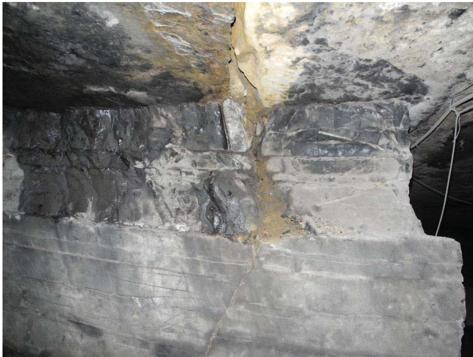
Figure 99: Example partly open and filled joint, pillar 3, photo nr.: 1413
