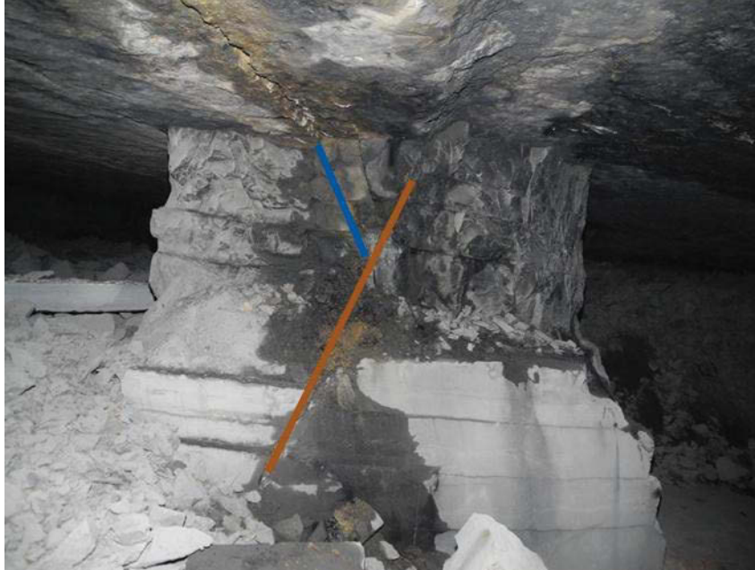
Figure 59: Pillar cut though by fault and joint
