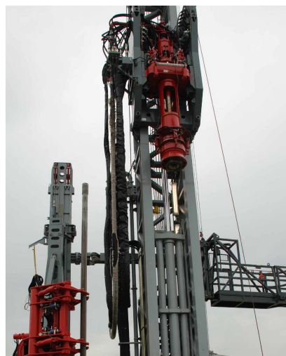
Figure 10: Hydraulic Hoisting System
