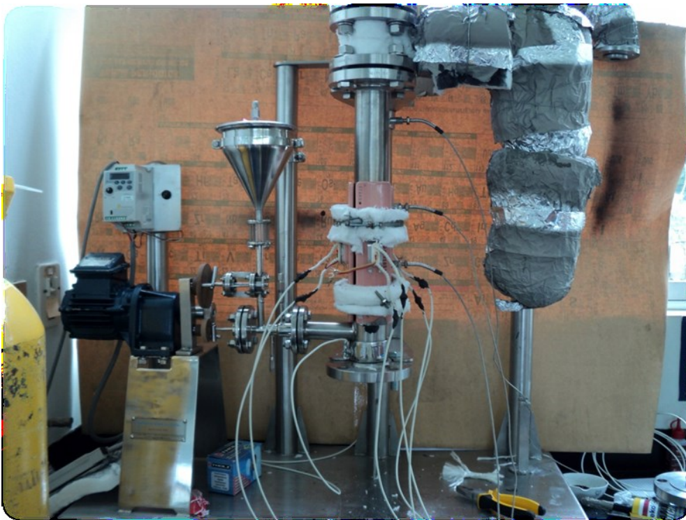
Figure 64: Installation of the heaters and the electric system in the PUCP-pyrolysis plant
