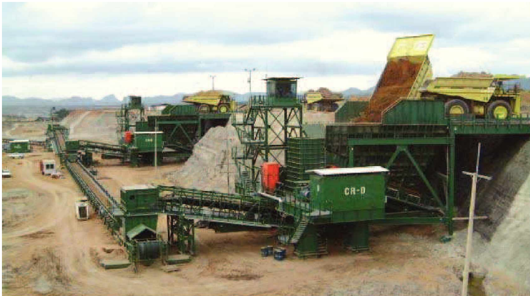
Fig. 3-36: MMD Semi mobile crushing unit
