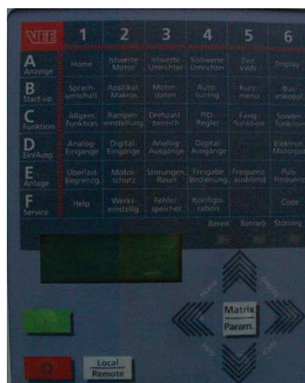
Photo 3.4-4 Control panel of the frequency converter for the roots pump flow control
