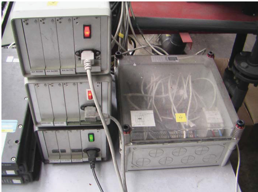
Photo 3.4-1 Power supply boxes
