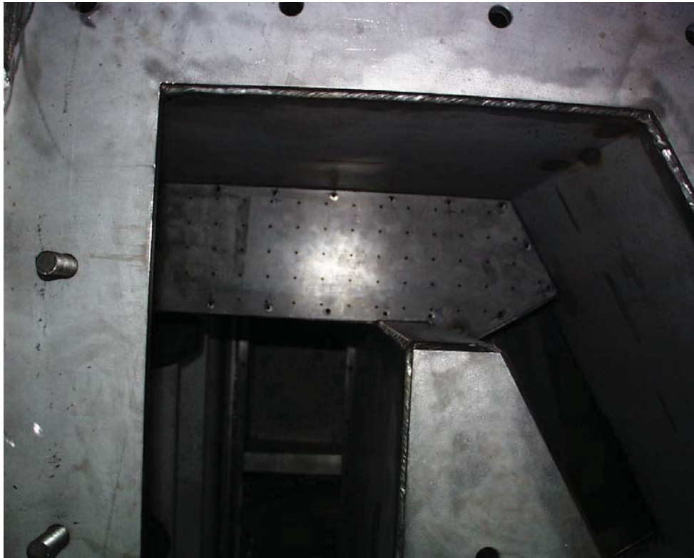
Photo 2.2-2 Delivering chamber for the bed material passage from the 2 nd heating chamber to the combustion chamber; the porous steel plate before mounting of steel screen on it
