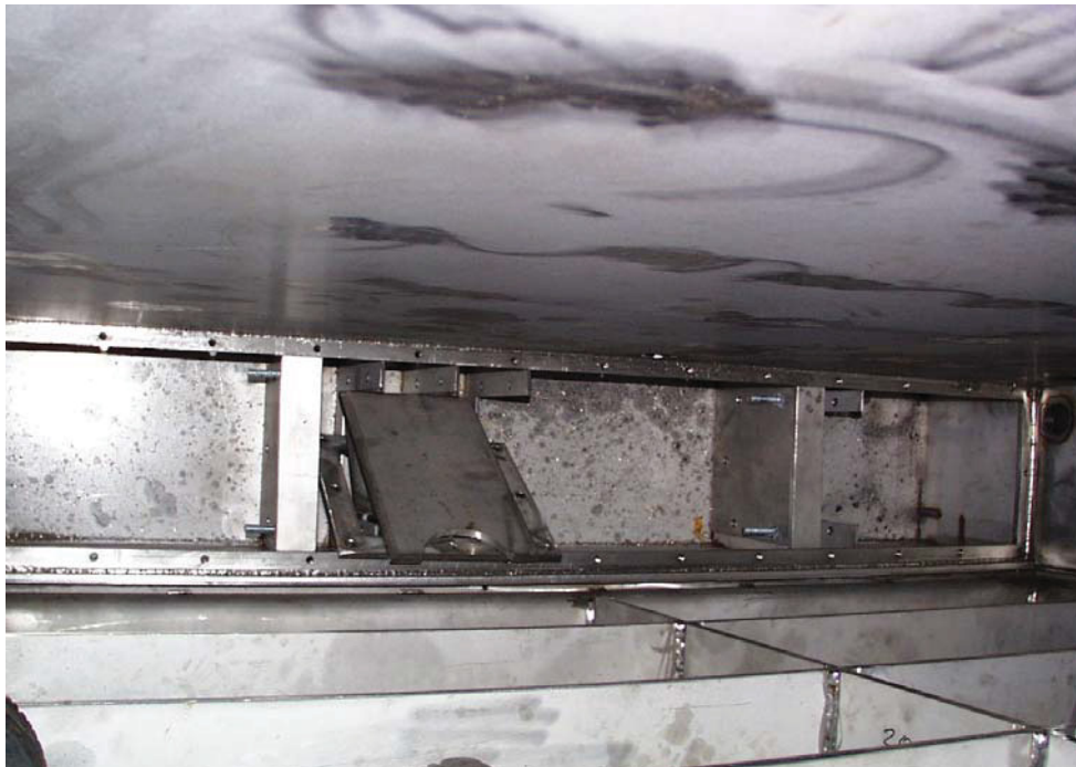
Photo 2.2-3 Wind boxes under the gas distributor in the FHE (The direction of view is vertically downward)
