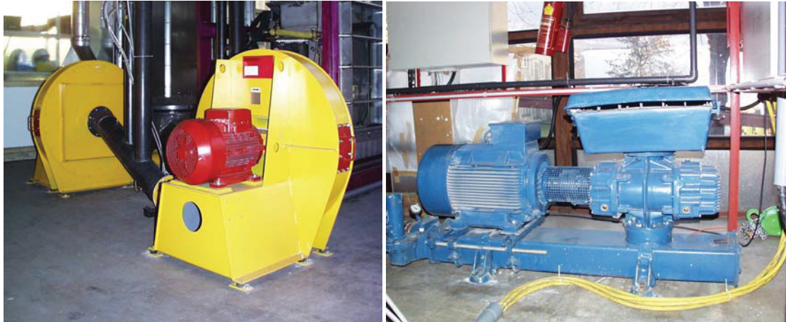
Photo 2.5-1 Ventilators (left) and roots pump (right)
