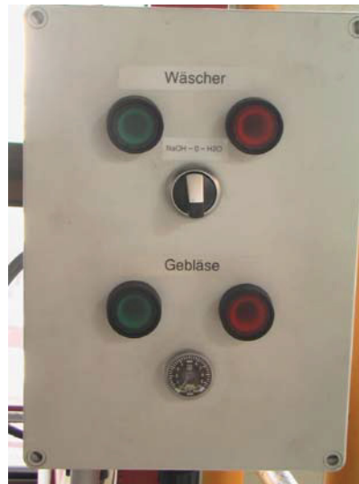
Photo 3.4-5 Controller for the ventilator in the air discharging system
