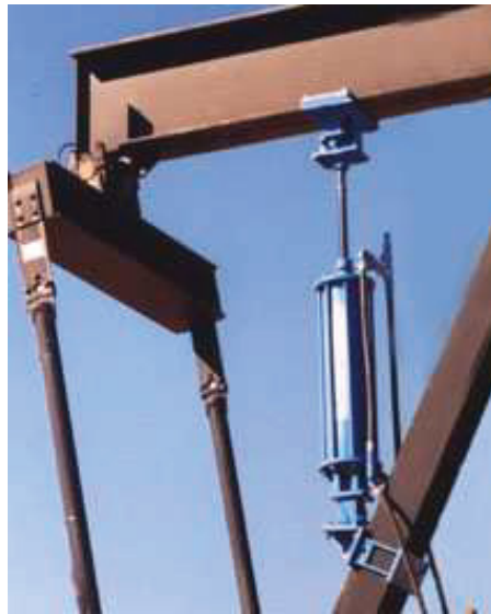
Figure 17: Conventional Unit with BMGC on a sampson post [21]
