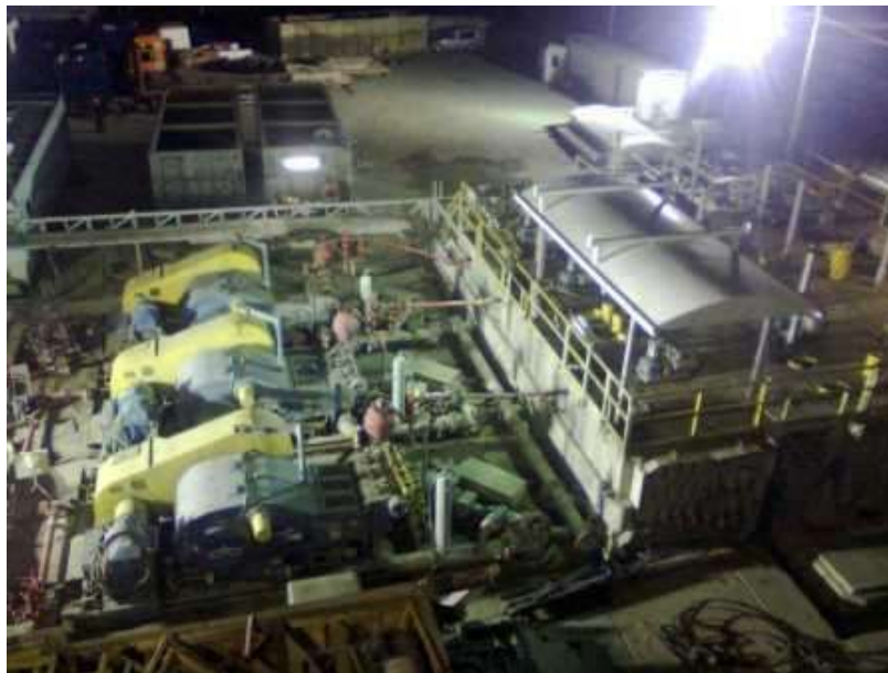
Figure 20: Mud pumps and mud tanks. Three mud pumps with 1600 HP each are used for a 500 t drilling rig.
