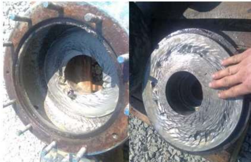
Figure 28: Erosion corrosion of a centrifugal pump housing. This picture was taken of a mud pump charging pump. The depth of the erosion corrosion is up to 15 mm. Almost the entire impeller was gone. The pump was changed after having changed the valves and pistons at the mud pump several times during drilling of the intermediate section. This led to slower drilling and subsequently to invisible lost time [33]. Permanent monitoring of the energy consumption of the charging pump would avoid this problem.
