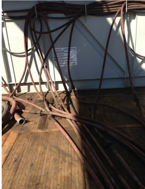
Fig. 26 – Accumulator hydraulic hoses.
