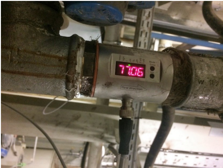
Figure 32: Flocculants dosage flow meter
