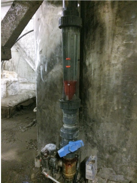
Figure 31: Newly implemented water flow meter
