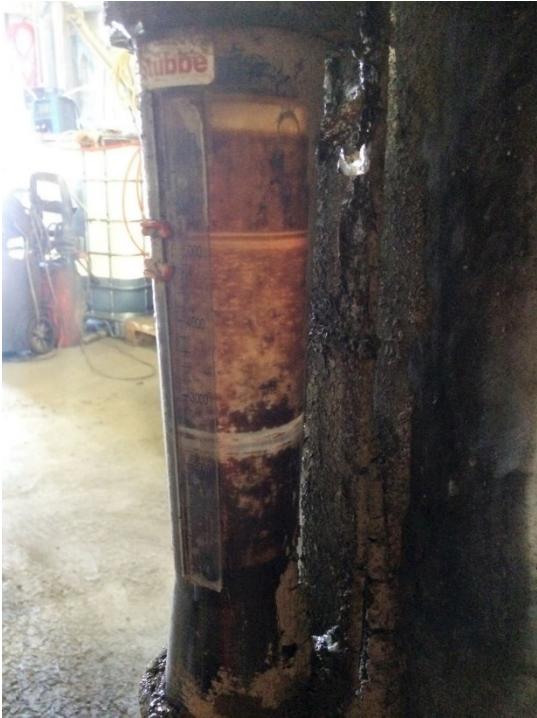
Figure 30: The dirty and damaged old flow meter
