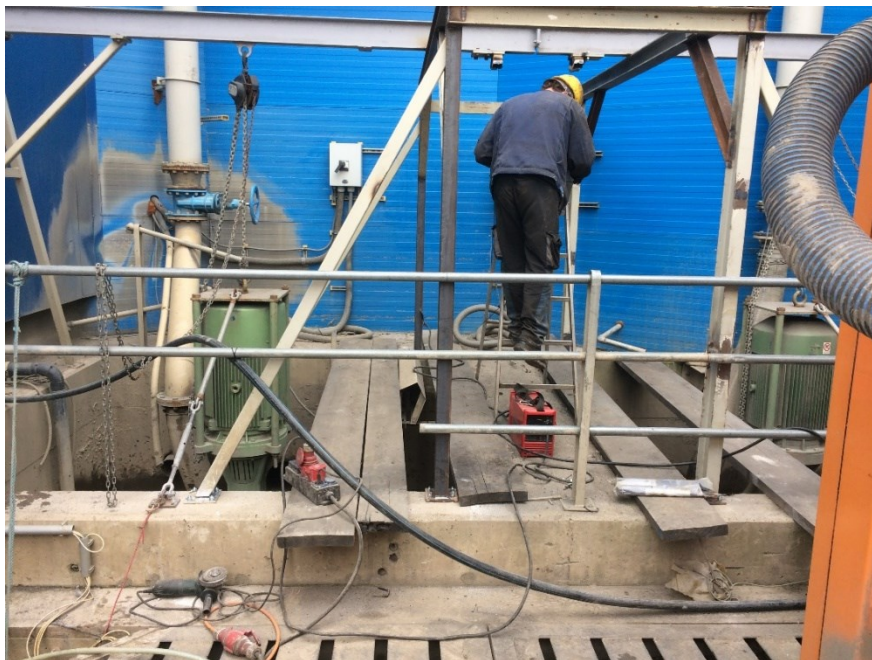
Figure 27: The two pump sumps with the separation in the middle
