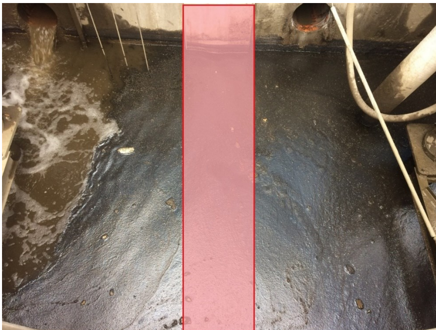
Figure 29: Top view on the basin already without wall. The red section is illustrating the removed wall
