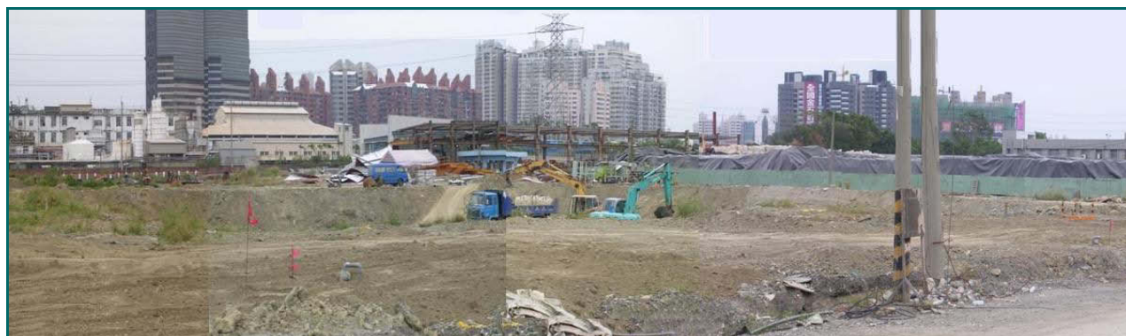
Figure 4-14: Panorama view of the former Formosa Chianjhen plant site in Kaosiung (industrial facilities demolished)
