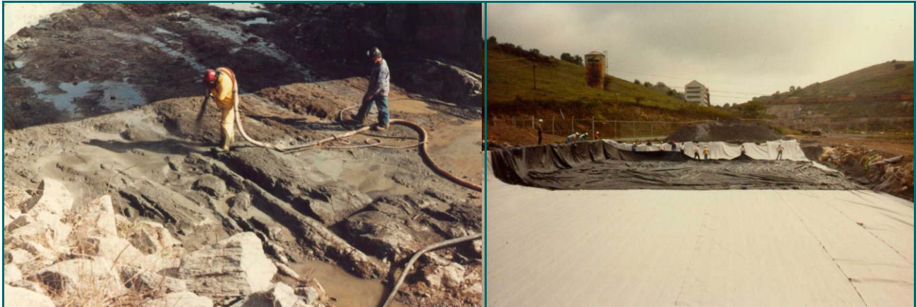
Figure 4-21: Capping activities performed at Saltville Waste Disposal Ponds 5 and 6 in 2001/02 (source: Golder Assoc.)
