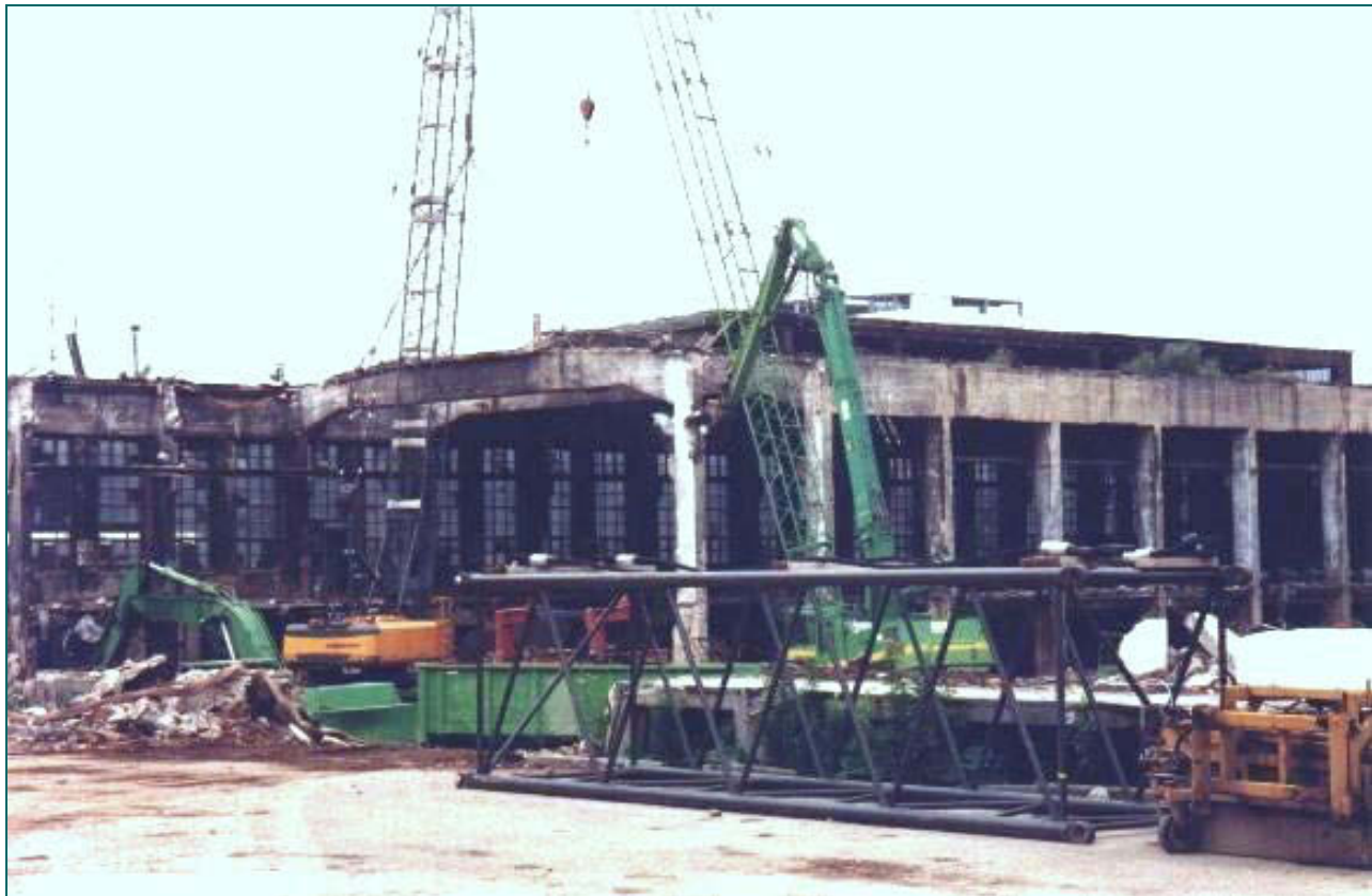
Figure 4-8: Demolition (controlled destruction) activities performed on chlorine plant I54 in Buna Schkopau in 2001
