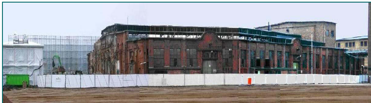
Figure 4-4: Chlorine-alkali electrolysis plant ‘Chlor III’ in Bitterfeld, East-Germany, built in 1917; closed in June 2000; demolished and dismantled in 2003 (40,000 tons of mercury-contaminated soil and rubble) xviii
