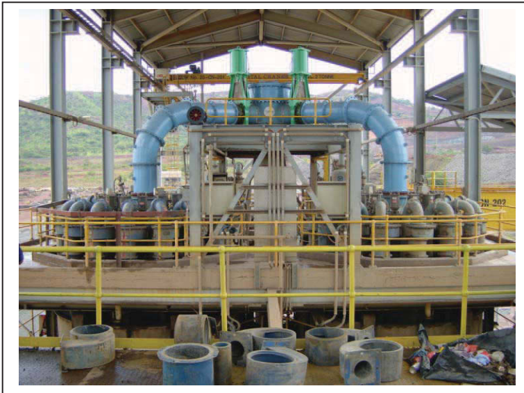
Figure 95: Geita Gold Mine, hydrocyclones, 2x16 units gMAX15, top fed by a central feed distributor, picture Roman van Ommen, 2008
