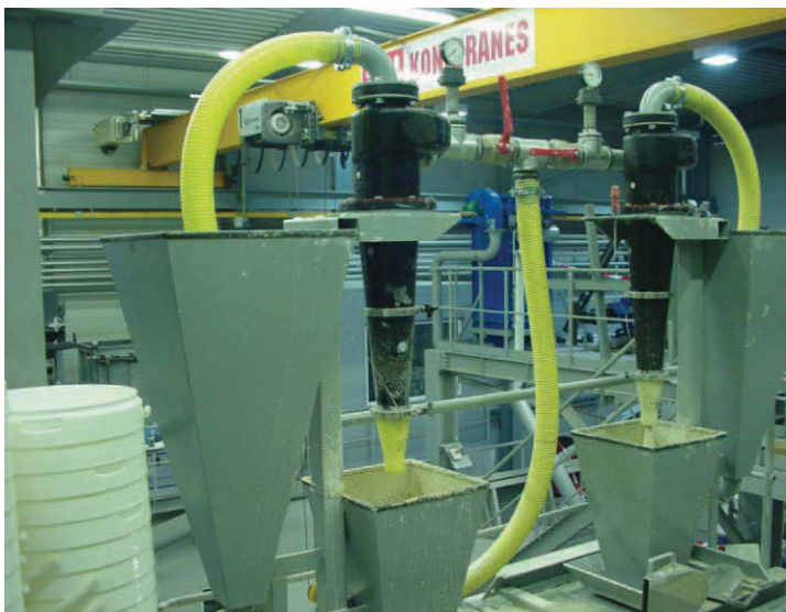
Figure 77: Hydrocyclones in test set up
