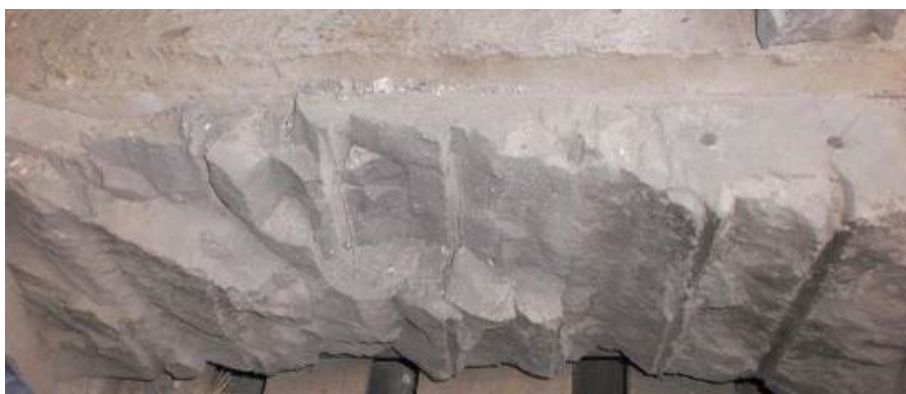
Figure 89: Extensive back breakage damage (B4R3, confined) (Petropoulos, 2011)
