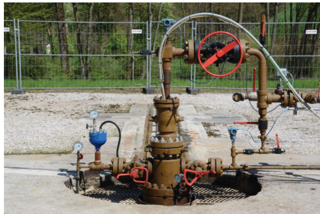
Fig. 7 – Surface installation of well V-030. The fluid level measurement device (painted blue) is mounted on the opened casing valve.
