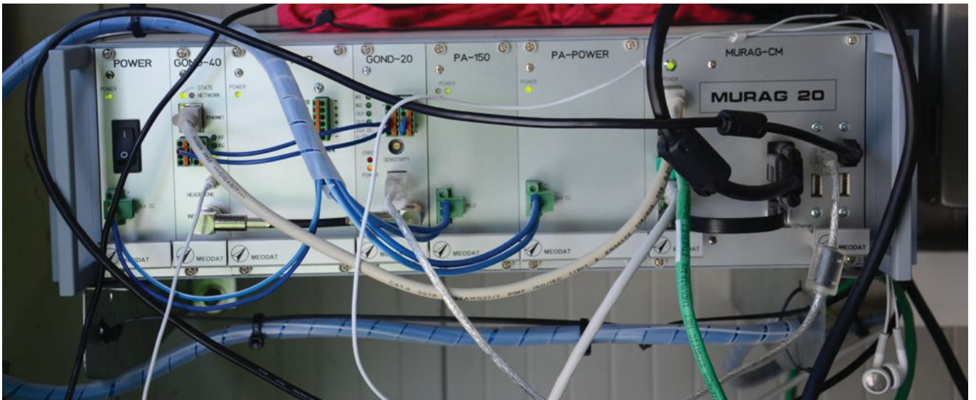
Fig. 4 – The Automated Fluid Level Evaluation Unit calculates the fluid level, stores it and feeds it into the SCADA system per standardized 4-20 mA interface for further processing.
