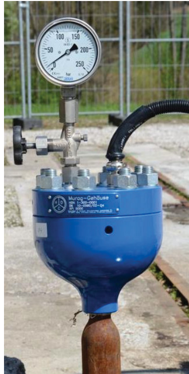
Fig. 3 – The Automated Fluid Level Measurement Device is mounted on the opened casing valve.
