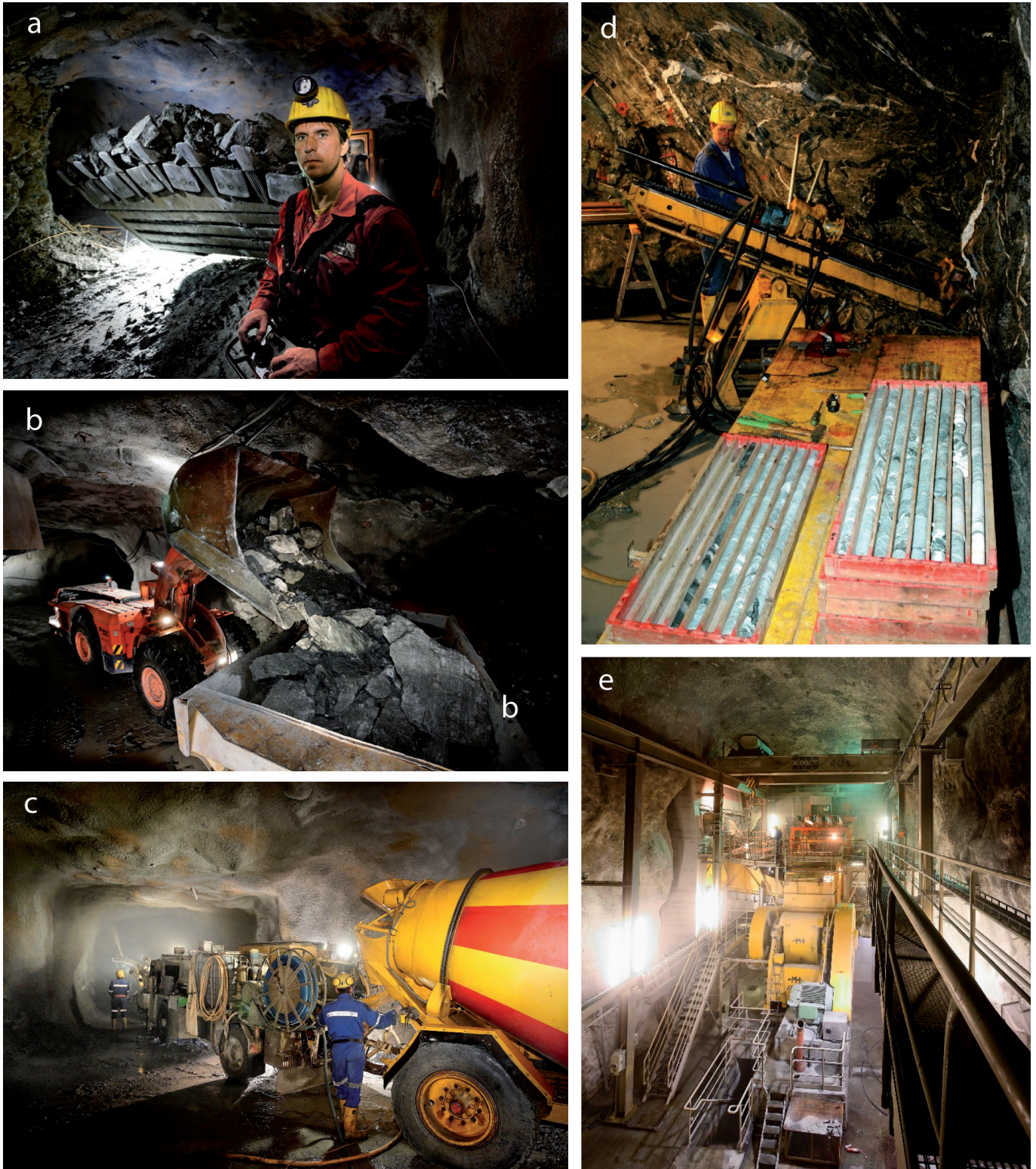
Fig. 18. a) Remote-controlled scooptram with 15 tonnes capacity. b) Mucking into an ADT truck for underground haulage from the lower sublevels. c) Shotcreting of development drifts. d) Underground diamond drilling. e) Primary jaw crusher in the underground crushing station.
