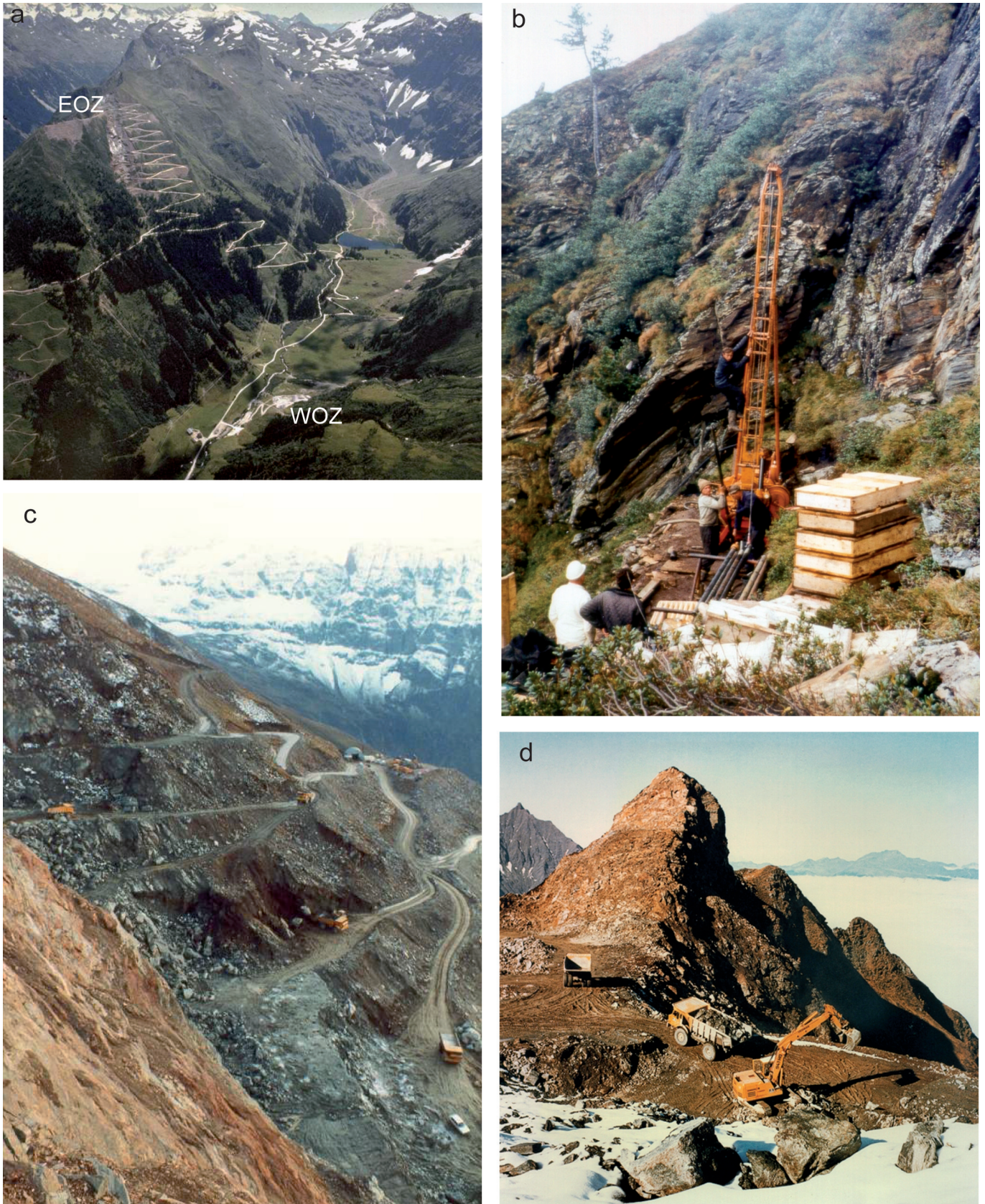
Fig 1. a) Location of the Eastern Ore Zone (EOZ, open pit) and Western Ore Zone (WOZ, underground) in the Felber Valley; view to ~S. b) Exploration drilling in the open pit area, 1972. c–d) Early mining operations in the open pit (mid-1970s). All photos from WBH archives.
